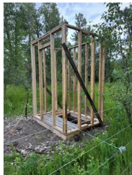
Outhouse in flood plain within 7.5m
